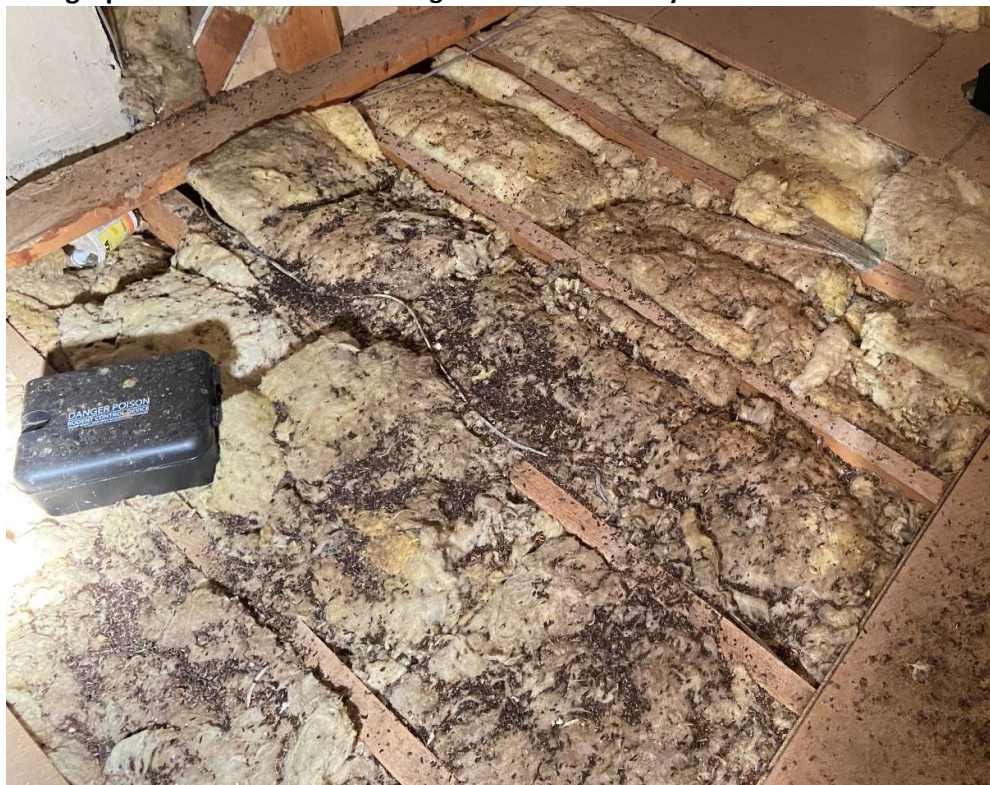
Photograph 1. Evidence of brown long-eared bat maternity roost at No2 Farnham Barn
